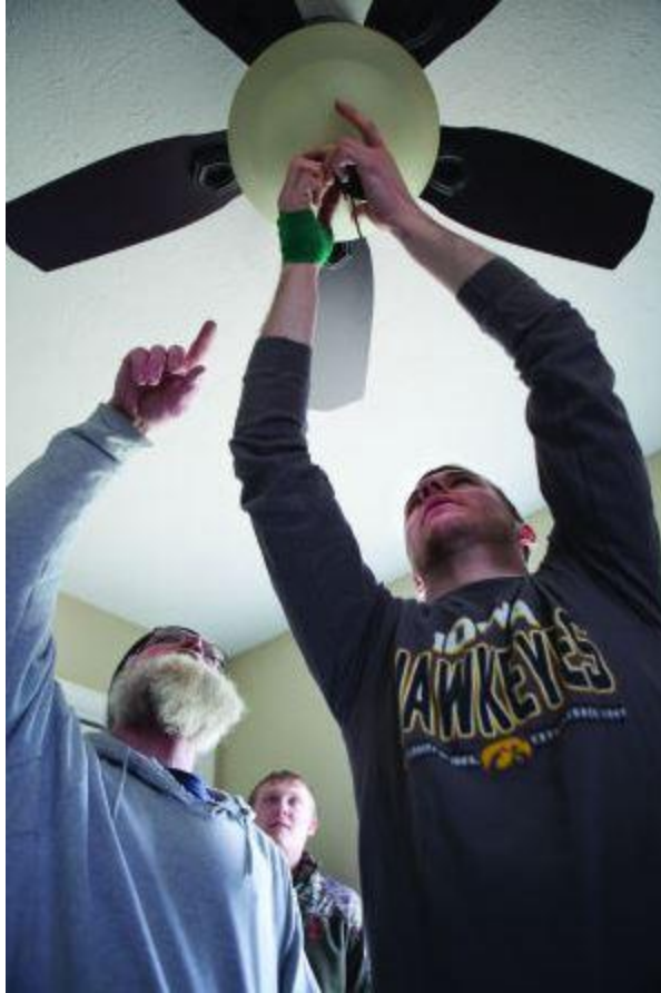
Electrical contractor Daryl Kirsch, left, speaks with an Iowa Western Community College construction technology class while student Zach Kahle puts the finishing touches on a ceiling fan the class installed March 27.
